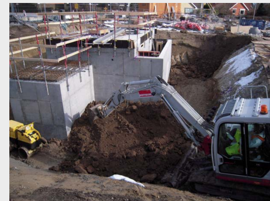
Pumping station in Taastrup, Denmark
